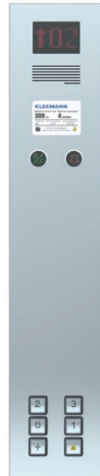
Car Operating Panel
